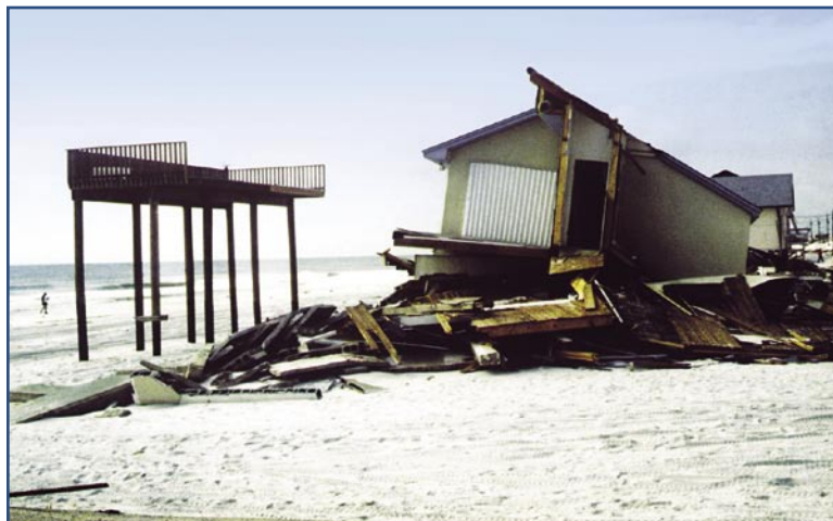
Damage from Hurricane Opal in Florida. This deck was designed to meet State of Florida Coastal Construction Control Line (CCCL) requirements. The house predated the CCCL and was not.
