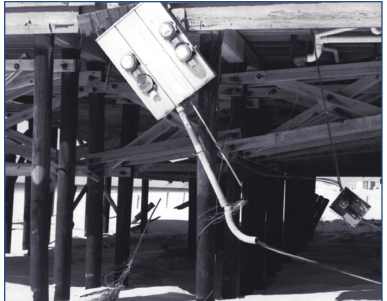
Electrical lines and box dislocated by hurricane forces.
