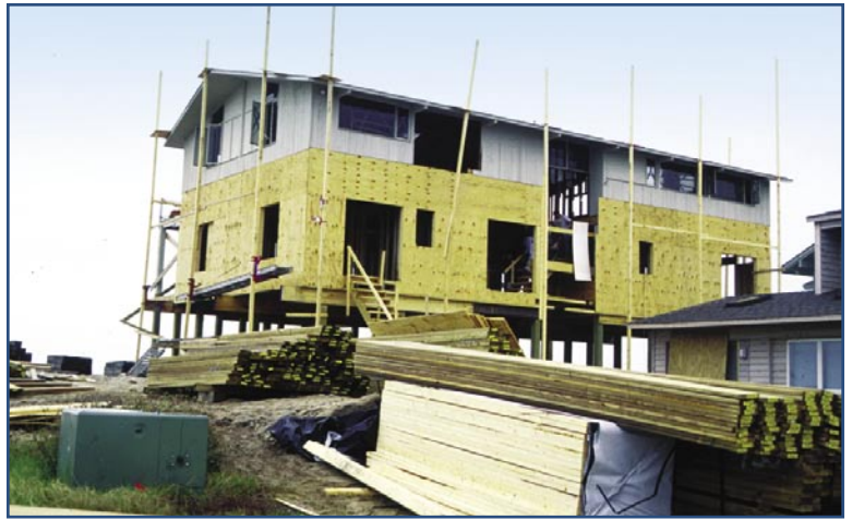
Figure 4 Vertical addition to a home damaged by Hurricane Fran. Pre-existing 1-story home became the second story of a home elevated to meet new foundation and floor elevation requirements.
