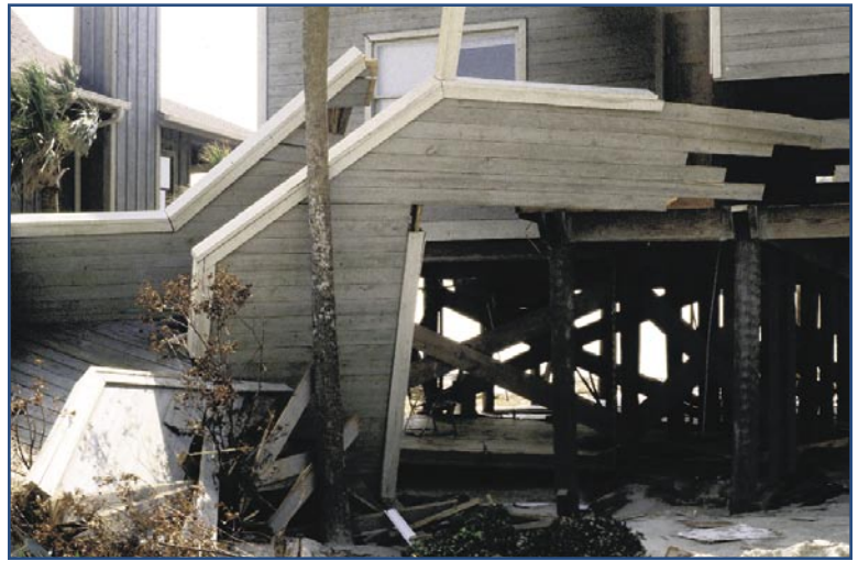
The rails on these stairs were enclosed with siding, presenting a greater obstacle to the flow of flood water and contributing to the flood damage shown here.
