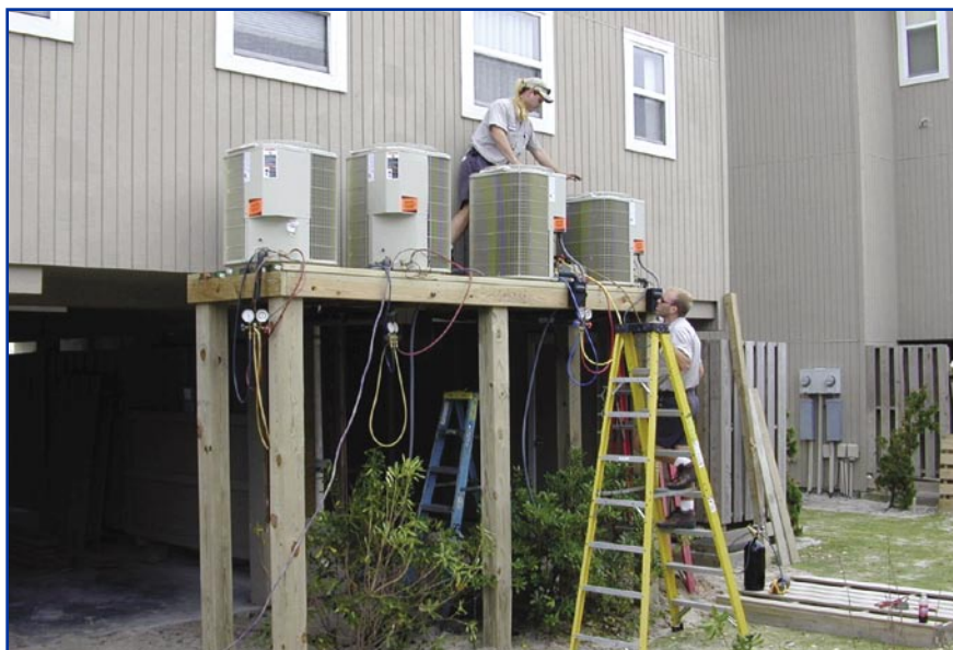
Elevated air conditioning compressors.
