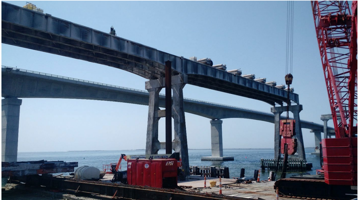
Figure 23 – Parapet segments in Span 146 had been removed (photographed on 4/7/2021)
