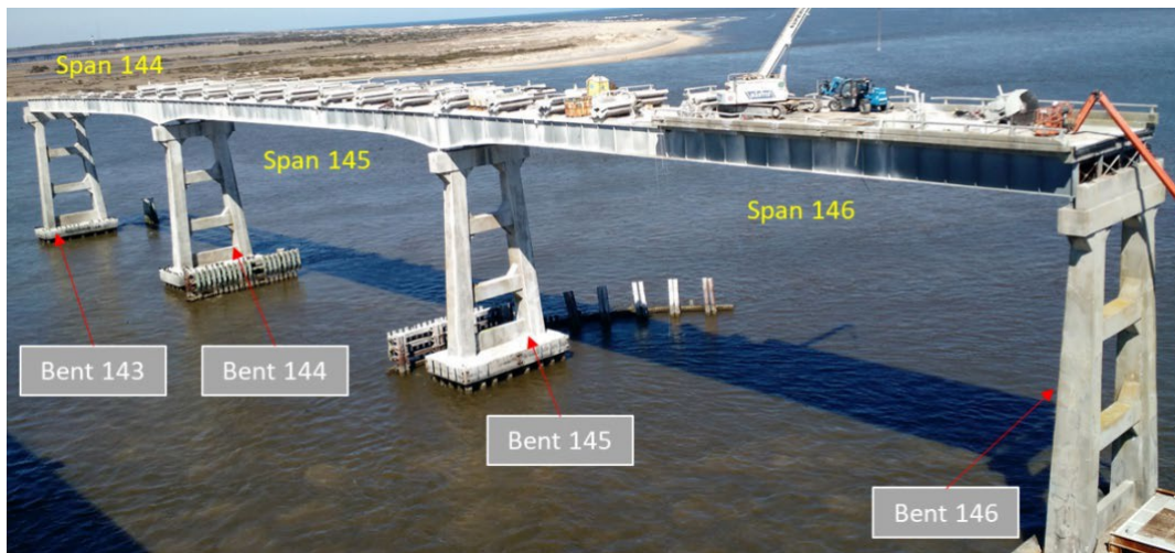
Figure 20 – Three steel girder spans under demolition – Looking north (photographed on 3/11/2021 by NCDOT)
