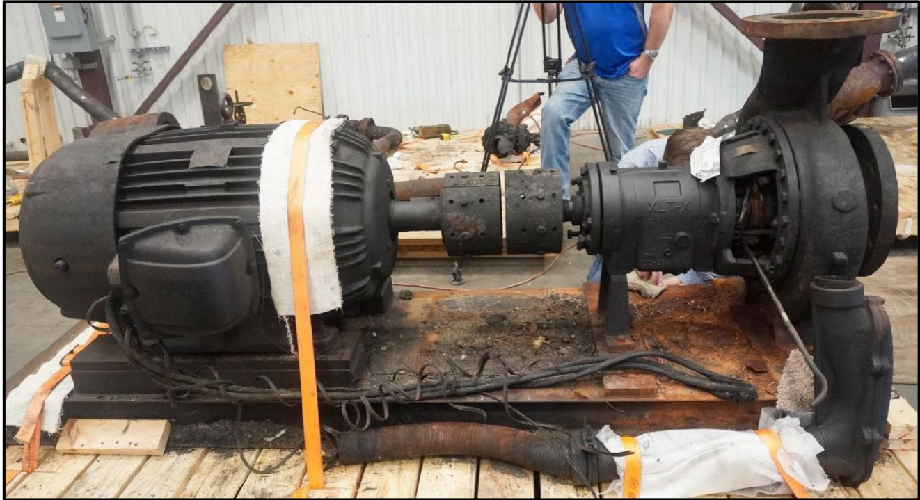
Figure 22. Tank 80-8 pump removed from ITC Deer Park terminal. Pictured is the pump kit on a pallet, as removed from the incident site. (Credit: CSB)
