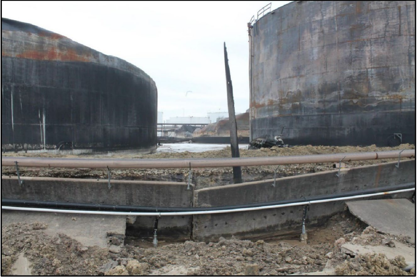
Figure 17. Close-up view of the First & Second 80's tank farm containment wall breach that occurred on Friday, March 22, 2019. (Credit: HCFMO).
