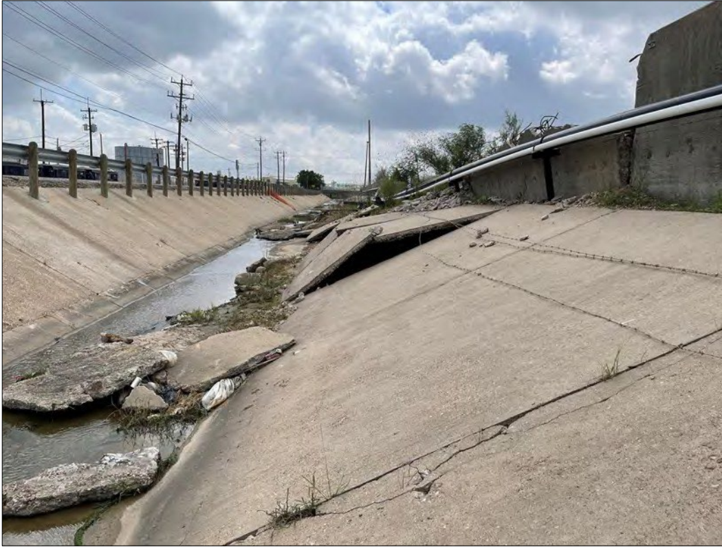
Photo 16: Damaged Section of Drainage Ditch, looking east
