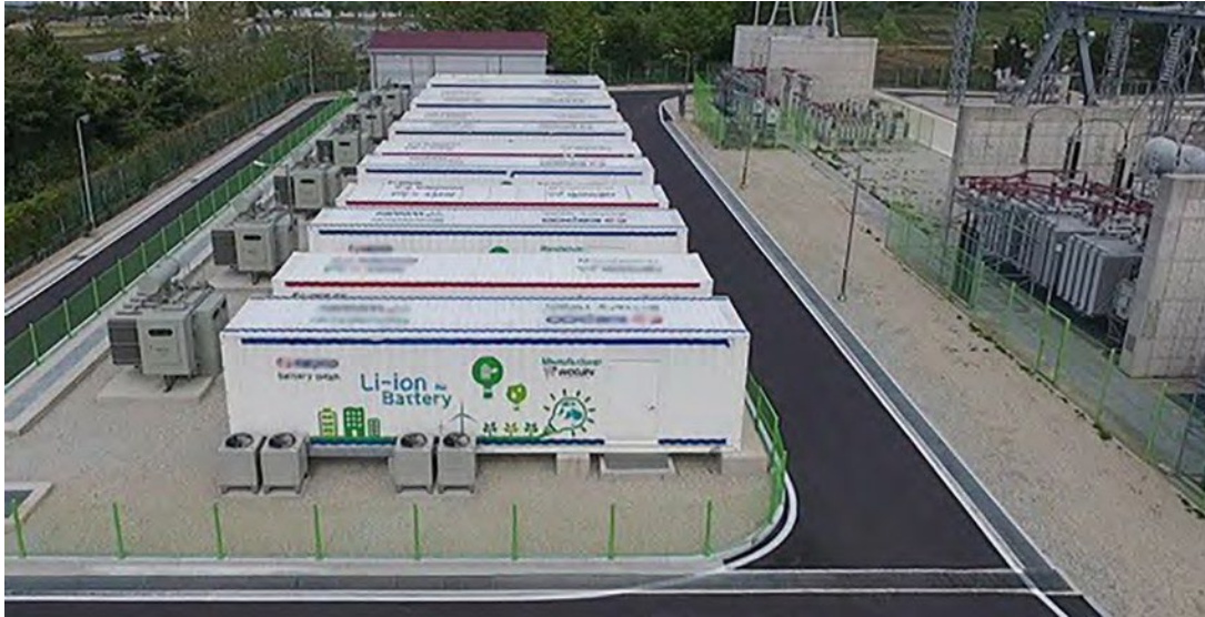
Figure D.4: Sokcho Battery Energy Storage System
