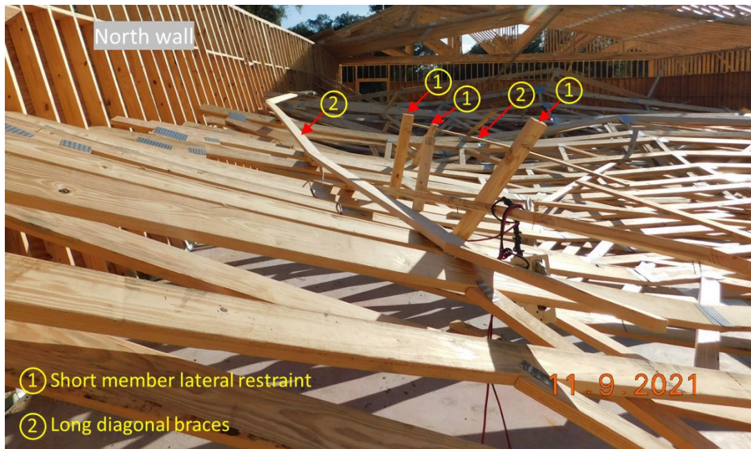
Figure 13 – Truss top chord braces at the north side after collapse – looking east
