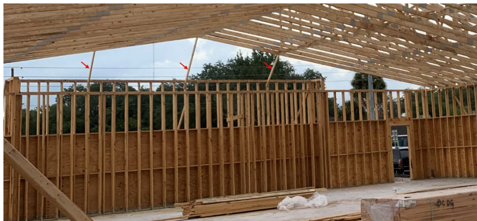
Figure 9 – Truss diagonal end braces at the west side – looking west (Photo by WW Build)
