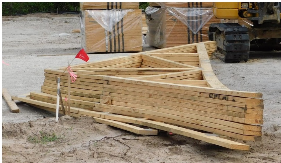
Figure 18 – Incorrect jobsite storage of trusses
