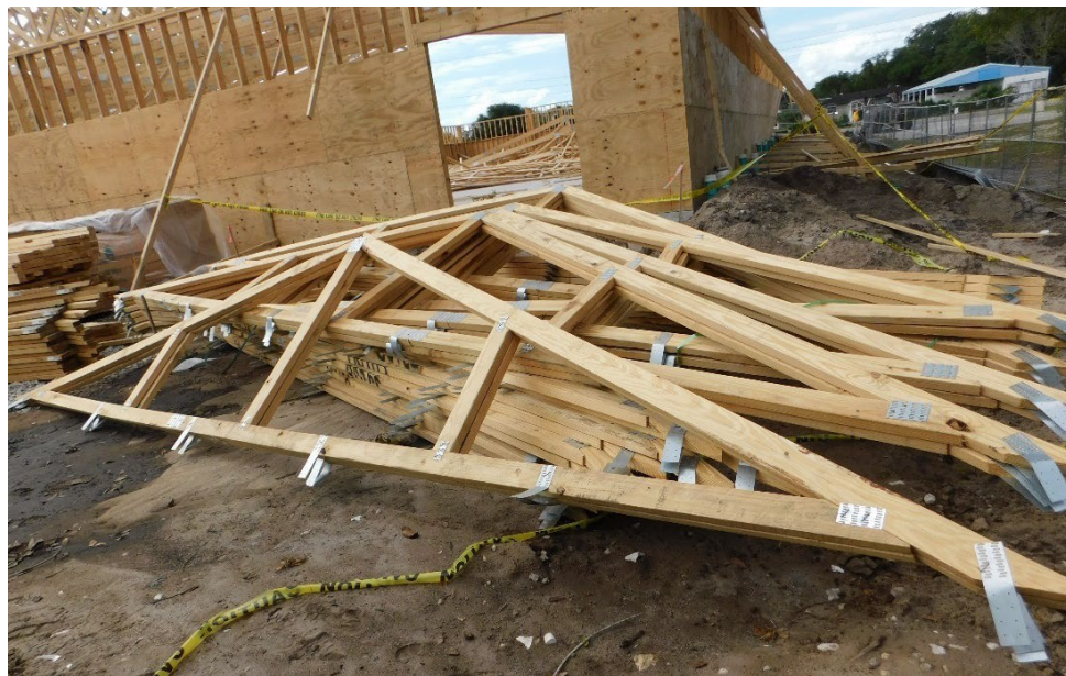
Figure 20 – Incorrect jobsite storage of trusses
