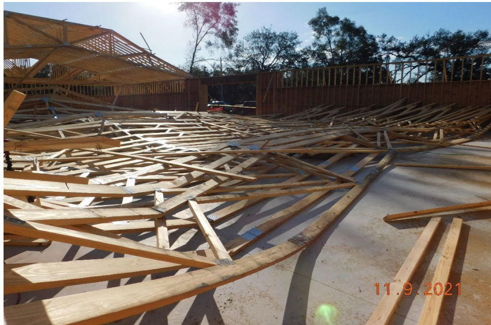
Figure 11 – Collapsed roof trusses – looking southeast
