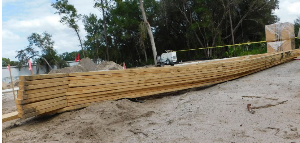
Figure 19 – Incorrect jobsite storage of trusses
