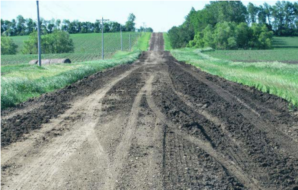
A road section heavily damaged during a wind energy construction project in wet conditions.
