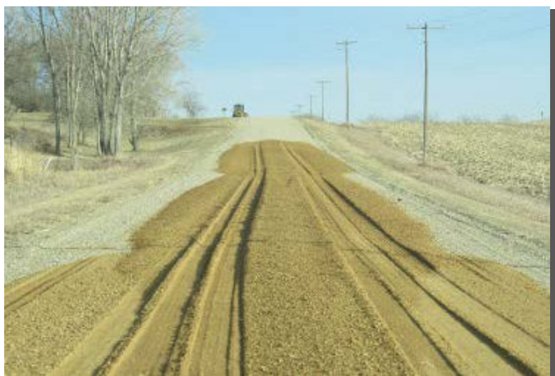
A good example of evenly dumping gravel on the road. Notice a grader is ready at the hilltop to begin processing the gravel.
