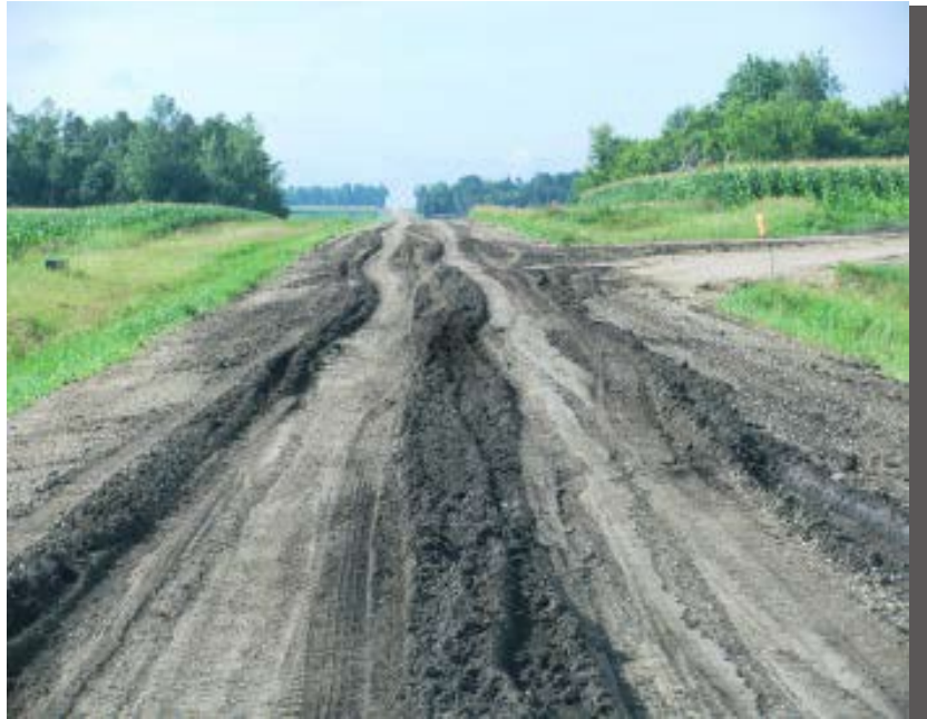
This road has been damaged by a heavy haul. Reshaping the entire road surface is required before new gravel is placed.
