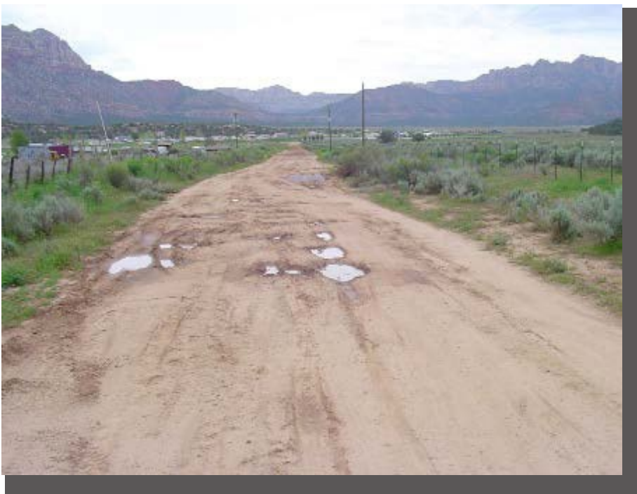
This road, located in a desert region, performs poorly even though the average annual precipitation is less than 10 inches per year.
