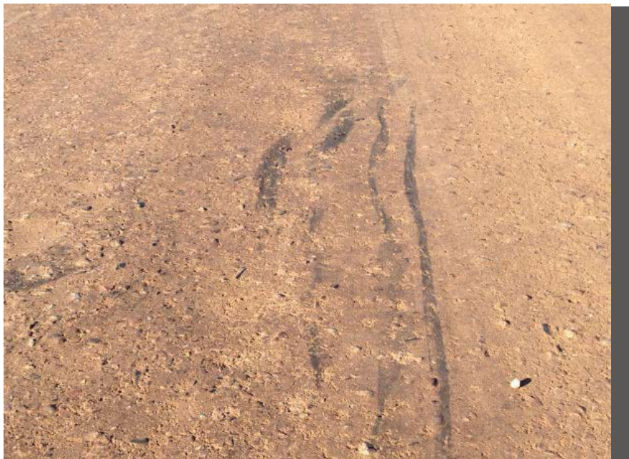
Outstanding record of performance on the same magnesium chloride stabilized road with a skid mark clearly evident.
