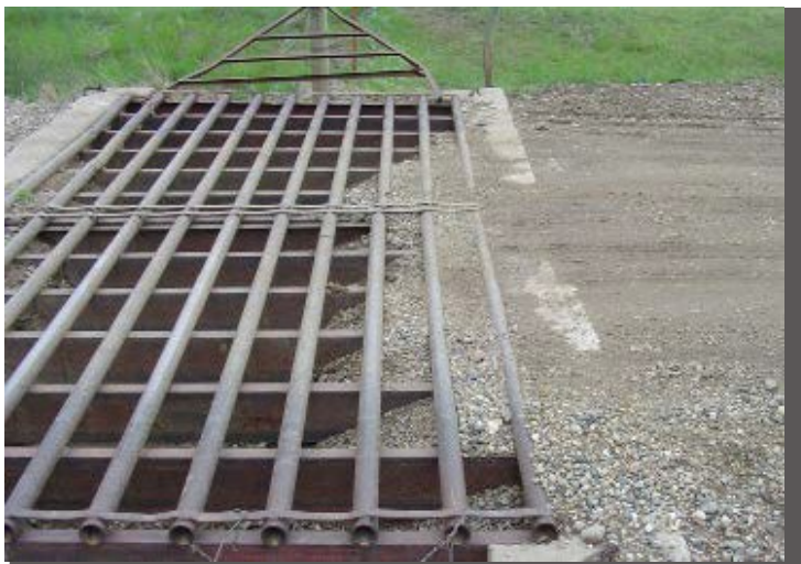
Care must be taken not to spill gravel into the cattle guard. Poor quality gravel with too much loose aggregate aggravates the problem of material spilling into the cavity spill gravel into the cattle guard.
