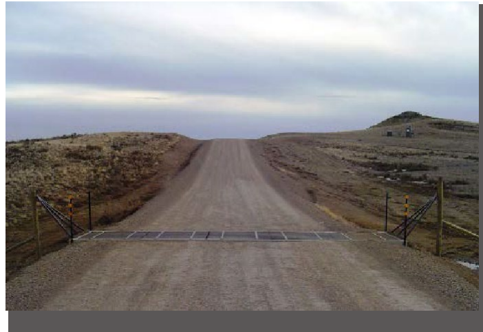
Road is shaped very well for a smooth crossing over the cattle guard.
