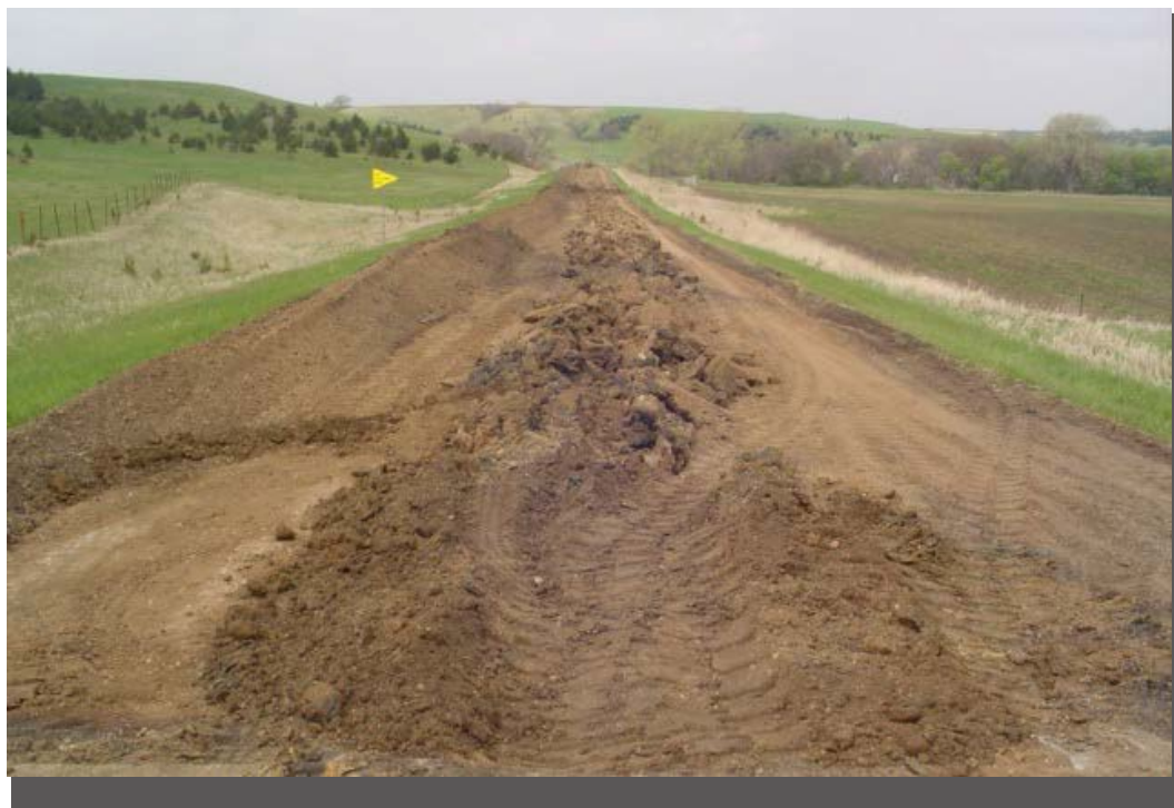
A road that had a constant problem with water percolating upward from springs beneath the surface. Work has just been completed to plow drainage pipe into the subgrade of this road.
