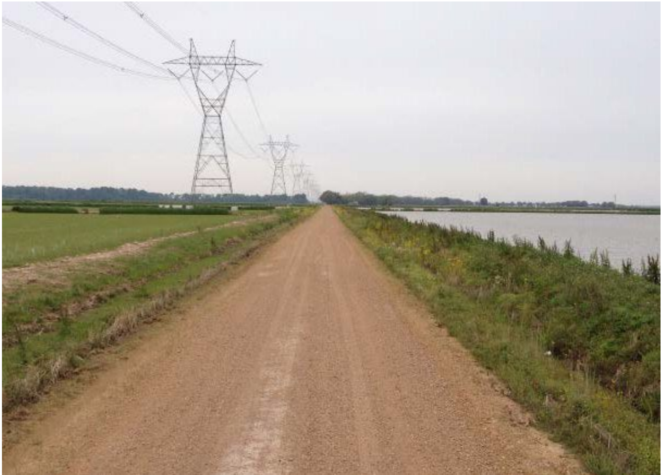
This road performs remarkably well because of good crown and good gravel quality in a very wet region.
