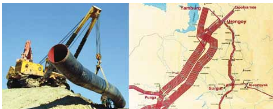
Fig. 3.11: From the laying of the Gazprom Bluestream pipeline (left). The pipeline is buried in a deep trench and leaves only a limited visual footprint once buried. The map to the right shows the incredible concentration of large diameter (56"; 1,40 meter diameter) pipelines in the Urengoy and Yamburg areas of northern Russia. This is part of the huge infrastructure of gas pipelines around the world. (Source: Gazprom)
