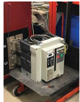
Primary Injection Testing
