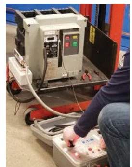
Secondary Injection Testing
