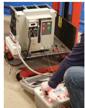
Secondary Injection Testing
