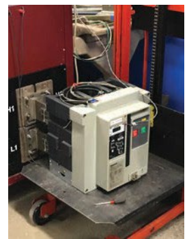
Primary Injection Testing
