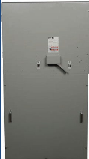
Main circuit breaker 3MFS1200RUG
